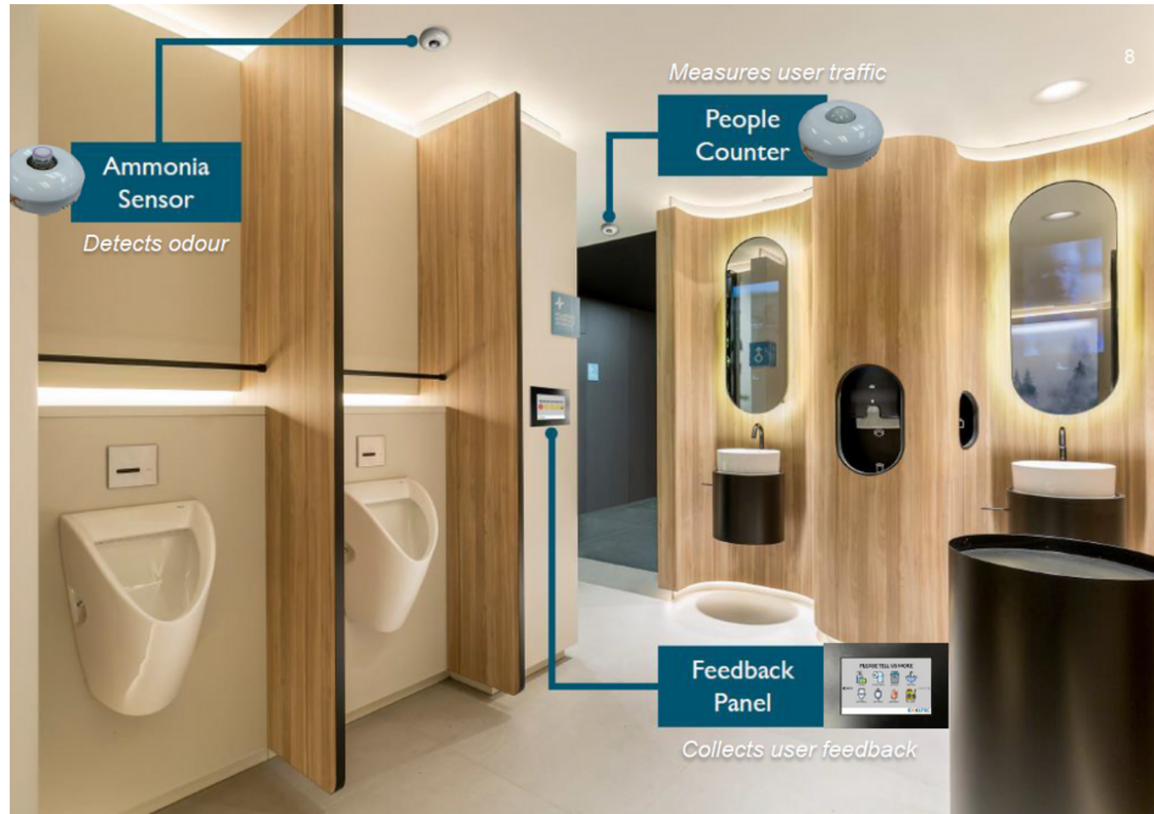
Smart Toilet, one of Exceltec's Smart FM Solutions
